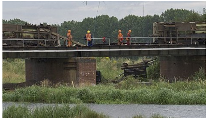
Fig. 2. The derailed wagons of freight train on Ely rail bridge [13]
