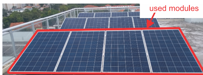
(a) Photovoltaic panels.
